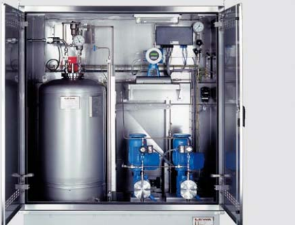
Flow proportional: precisely controlled odourant addition e. g. in the natural gas supply
