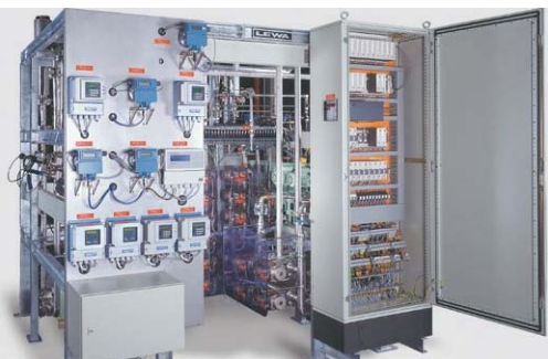
... individually designed metering packages are optimally matched to each other
