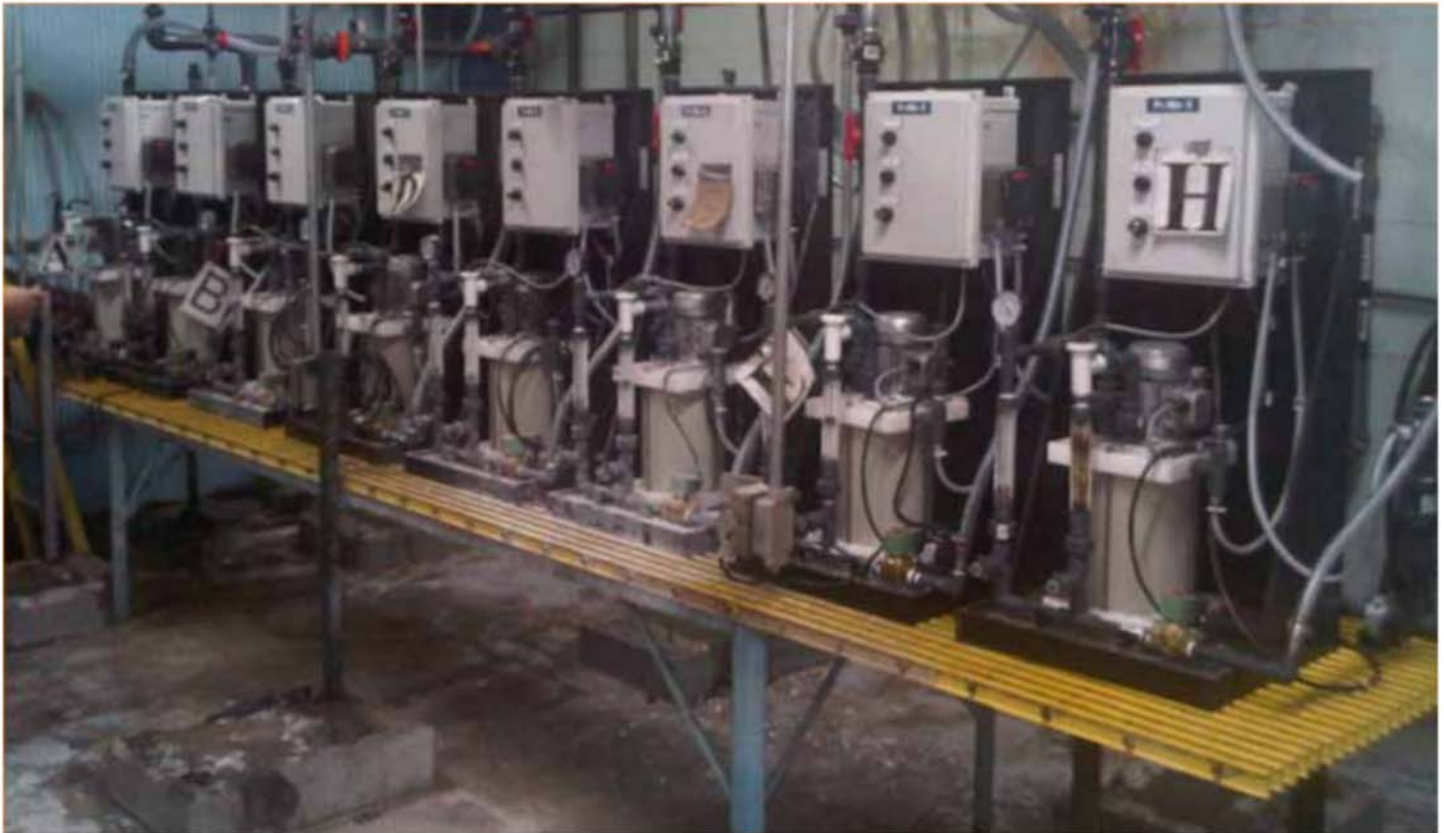
2010 completed installation and operational ProMix-S units.
