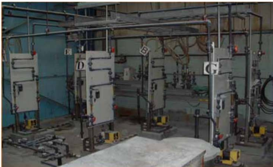
2001 Polymer Make-down utilizing LMI pumps and static mixers. The LMI pumps were replaced in 2002 with ProMinent Sigma 1 Control series pumps; control improved immediately.
