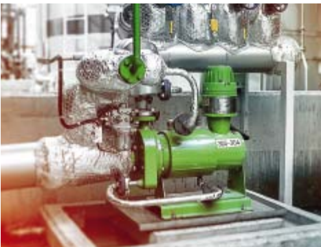
High melting point type pump in a chemical plant.
