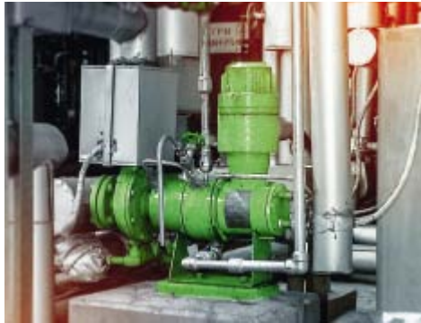
High-temperature type pump in a chemical plant.
