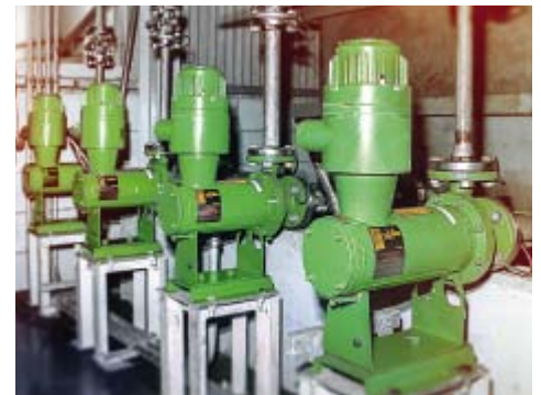
Basic type pumps in a chemical plant.
