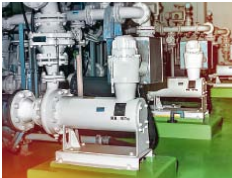
Basic type pumps in a water treatment plant. (Titanium casing & impeller)
