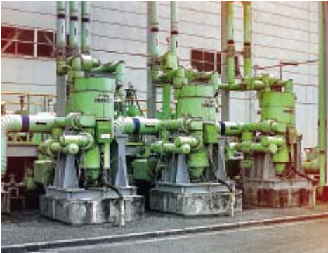
Reverse circulation type pumps for pumping LNG as Cooling medium. (Vertical type, Motor output 75kw)
